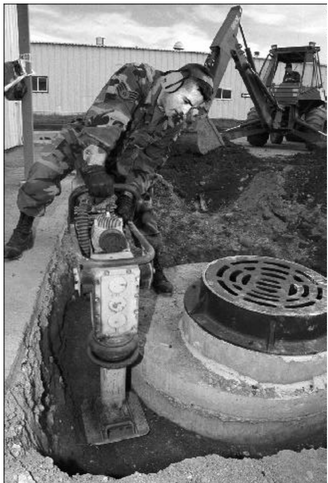
Staff Sgt. Steven Romine flattens the ground around the new storm drain catch basin outside the flight line facility.
