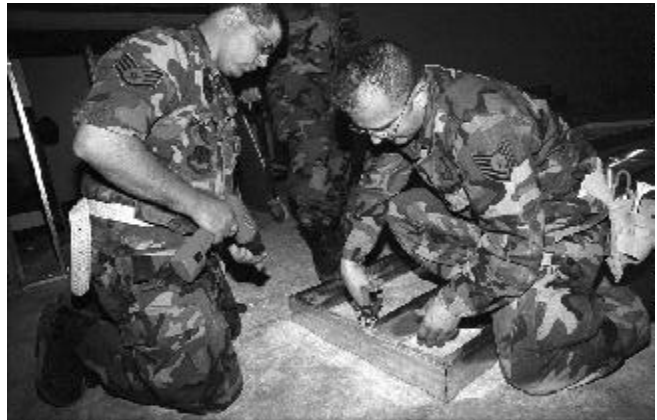
Staff Sgt. Mark Sparagna (left) and Tech. Sgt. Edwin Reyes (right) prepare a stud wall for the 210th Rescue Squadron communications and control room.
