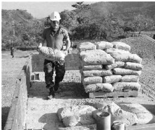
Spc. Mark Leonard loading cement bags for a construction site. Photo by Col. John Dwyer, PAO, DMAVA.
