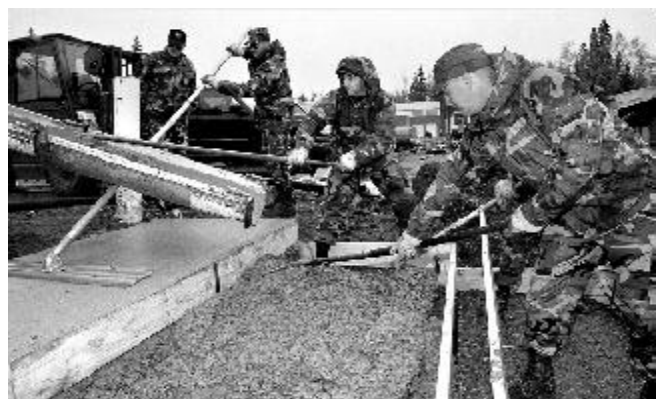
Civil Engineering Squadron members pour the concrete for the steps behind the operations building at Kulis Air National Guard Base.
