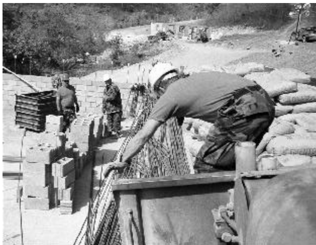
Two hours and 14 miles later the supplies are dropped off at the construction site. Photo by Col. John Dwyer, PAO, NJDMAVA.
